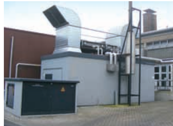
Acoustic enclosure (concrete construction)
