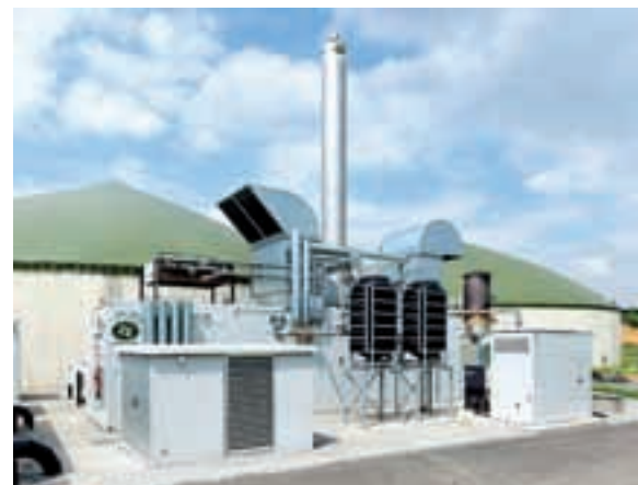
Containerised CHP, ready for connection
