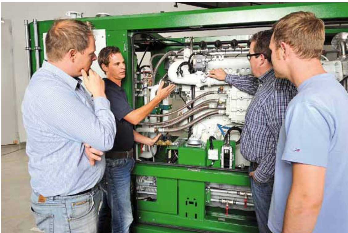
Inspecting, maintaining, and rectifying faults in combined heat and power units are the focus of the practical 2G service training programs.
